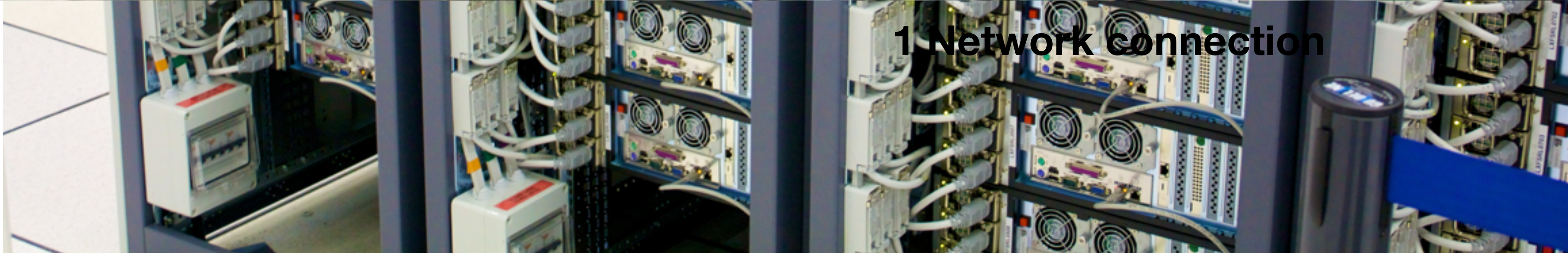
Systematic power distribution; 3 power supplies; 2 fans; 1 network connection
