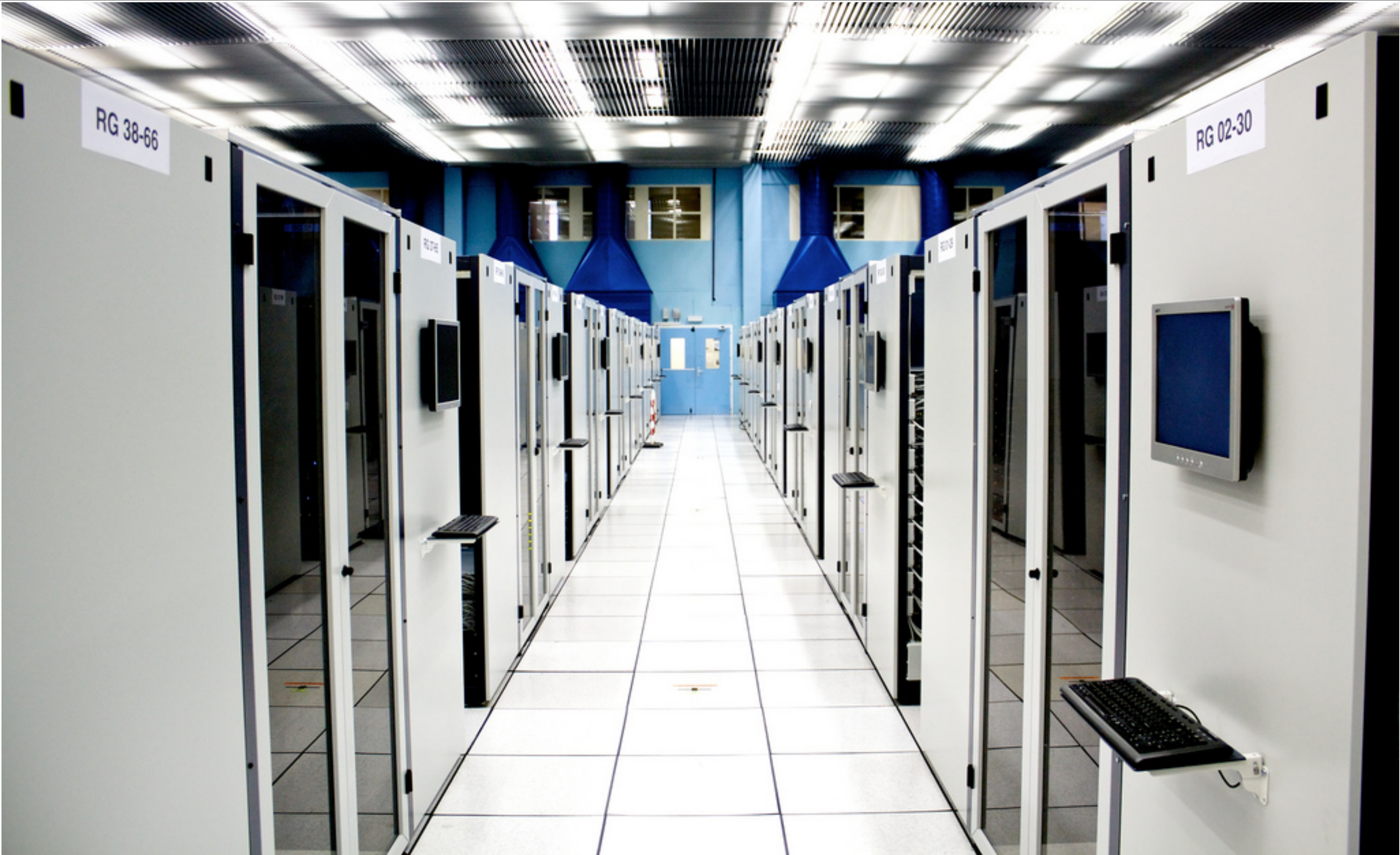
Typical machine room
